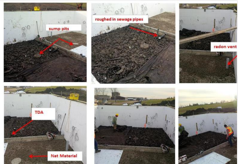
placing TDA in the southern half and natural material on the northern half of the ground
