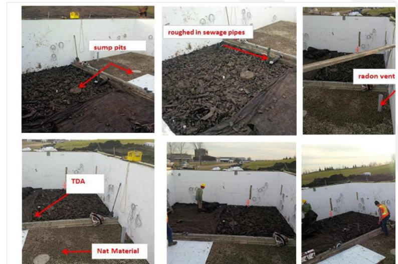
placing TDA in the southern half and natural material on the northern half of the ground
